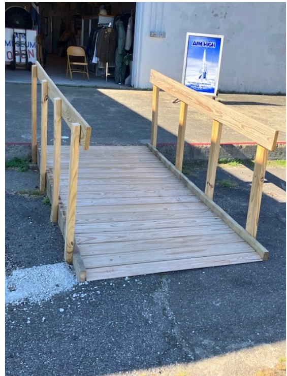
Many thanks to Les Shaw for building this new ramp leading to the Museum's entrance
